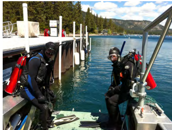
Research divers Brant Allen and Katie Webb preparing to lay the first section of the underwater cable for Tahoe's first real-time water quality monitoring station.
