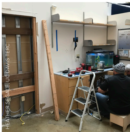
Science Center Equipment Updates began by removing the old monitors and video equipment
